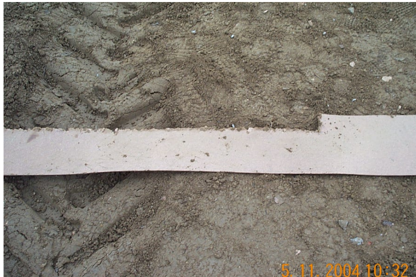
Figure 20 – Damaged fiberboard on the topsoil lane
